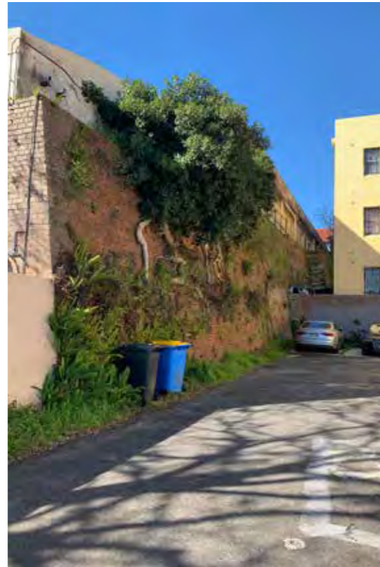
Northern Interface: blank brick retaining wall to loading dock and car parking of 3 Darling Point Road - Ranelagh Tower
