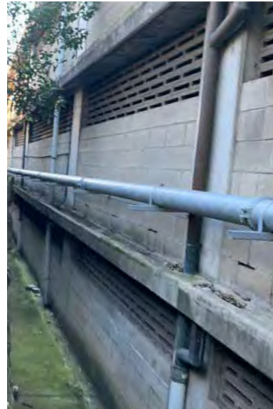
Northern Interface: concrete & block wall to loading 3 storey + roof deck podium car parking of 3 Darling Point Road - Ranelagh Tower
